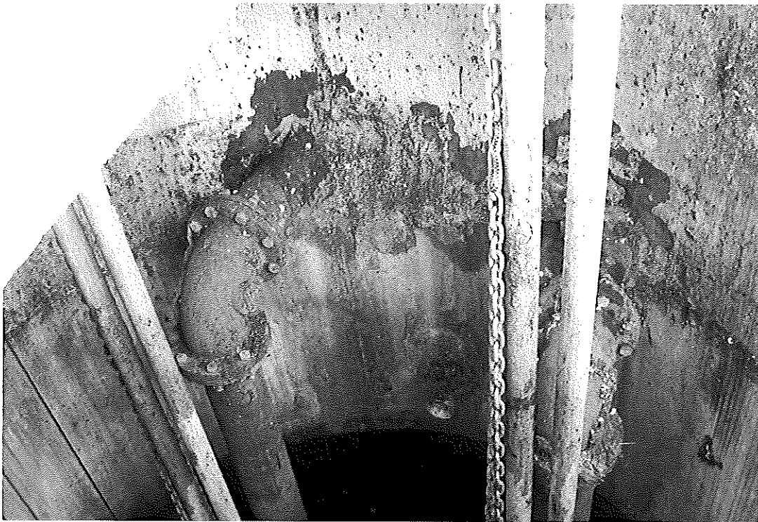
Figure 18. Main Lift Station Wet Well
