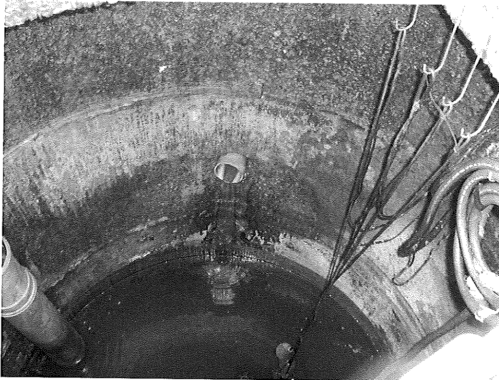
Figure 13. Interior of Golf Course Lift Station
