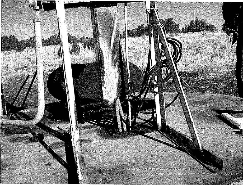
Figure 8. Exterior of Lift Station 5B-2
