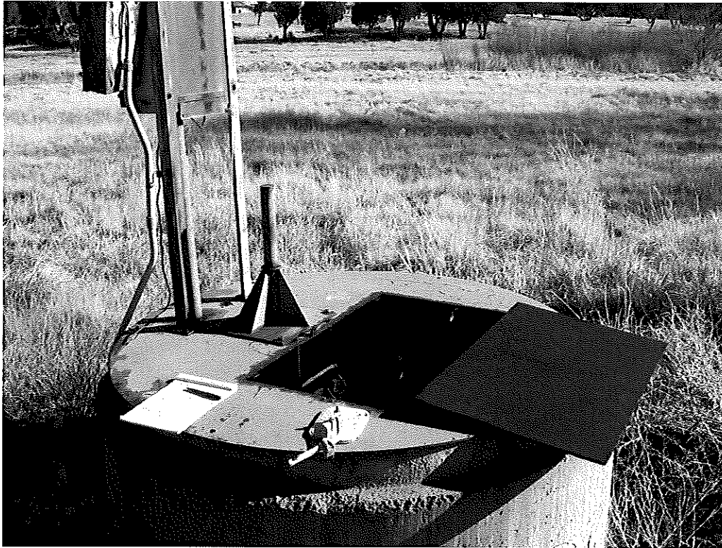
Figure 15. Exterior of Motel Lift Station
