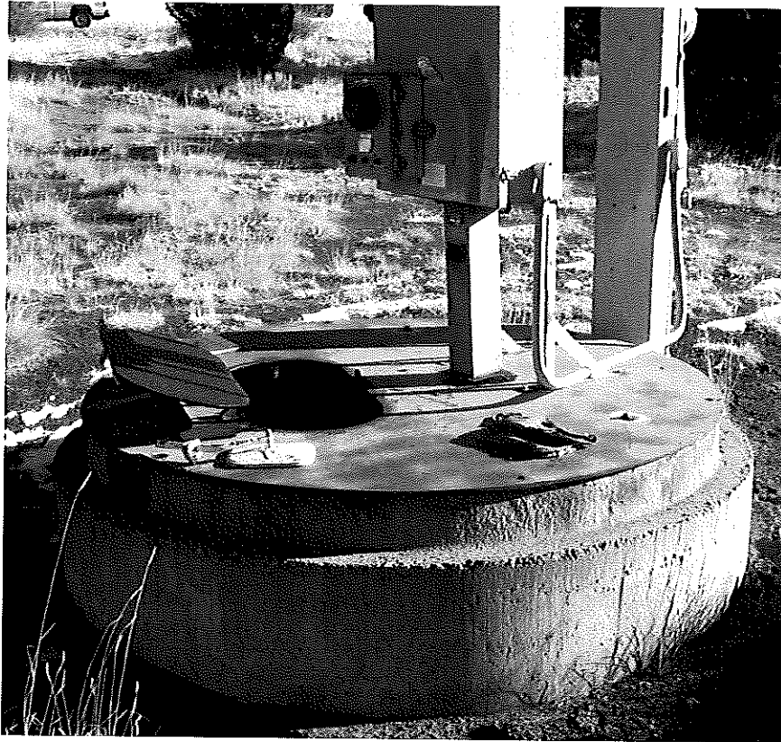
Figure 5. Exterior of Lift Station 5B-1
