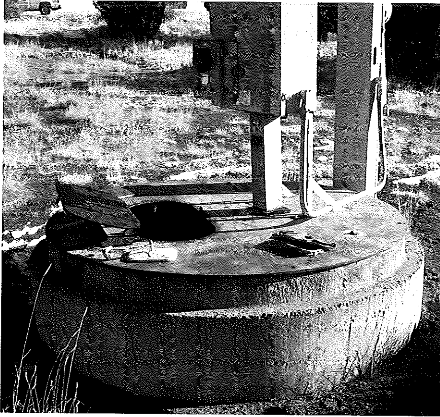
Figure 5. Exterior of Lift Station 5B-1
