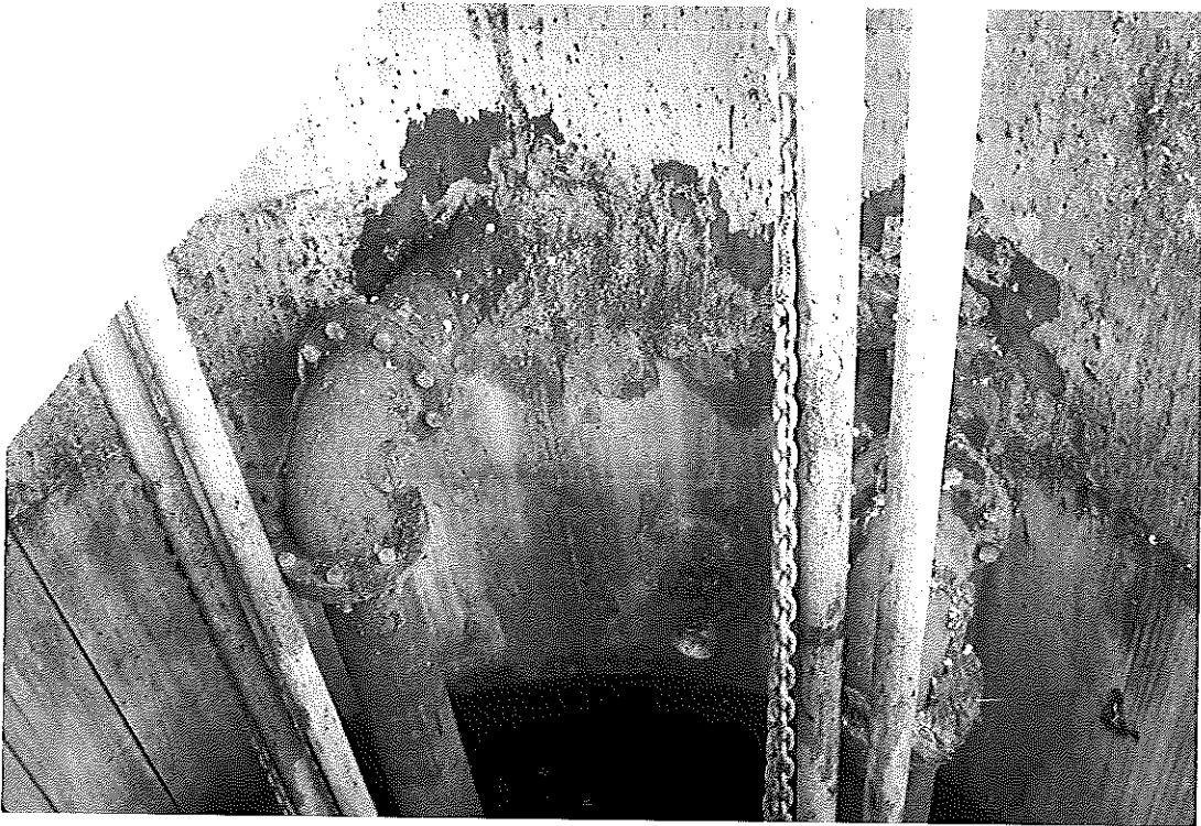
Figure 18. Main Lift Station Wet Well
