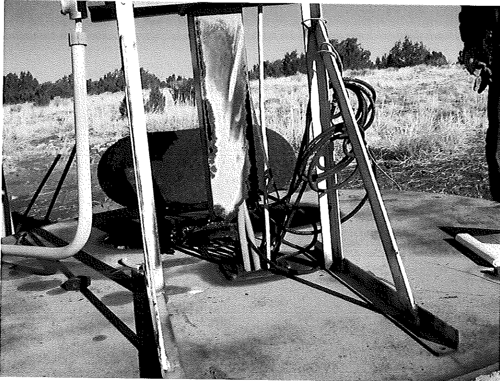
Figure 8. Exterior of Lift Station 5B-2
